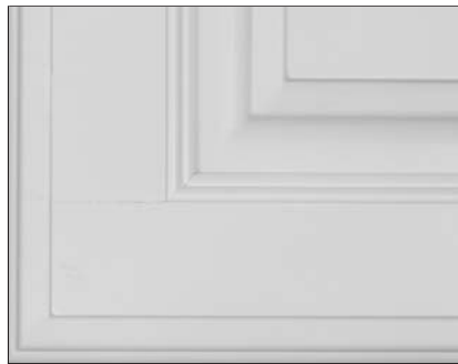
Example of door front joint separation
