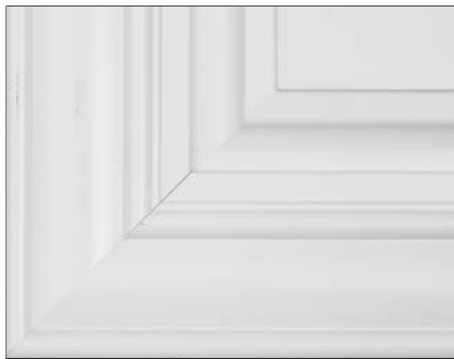
Example of door front joint separation
